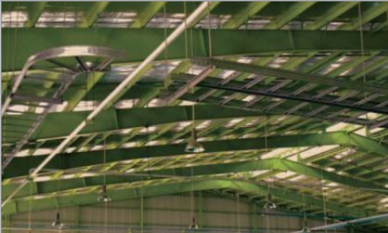
INSTALLATION LIGHTING AREA FACTORY
