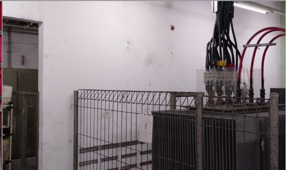
INSTALLATION CABLE TRAF0 2000 KVA
