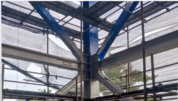
PAINTING STRUCTURE CORROSIVE
