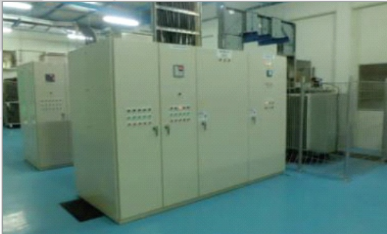
INSTALLATION LV MDB, BUS DUCT, TRANSFORMER
