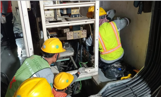
INSTALLATION CABLE TRAF0 2000 KVA
