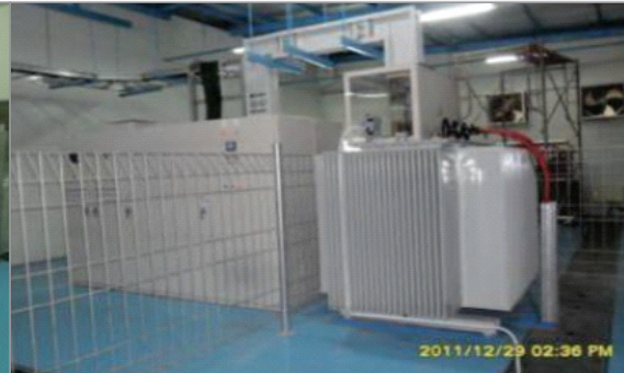
INSTALLATION LV MDB, BUS DUCT, TRANSFORMER
