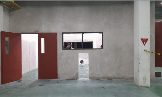
BUILDING MAINTENANCE ROOM
