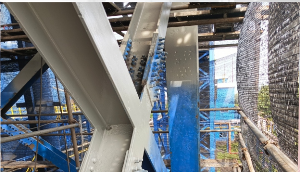
PAINTING STRUCTURE CORROSIVE
