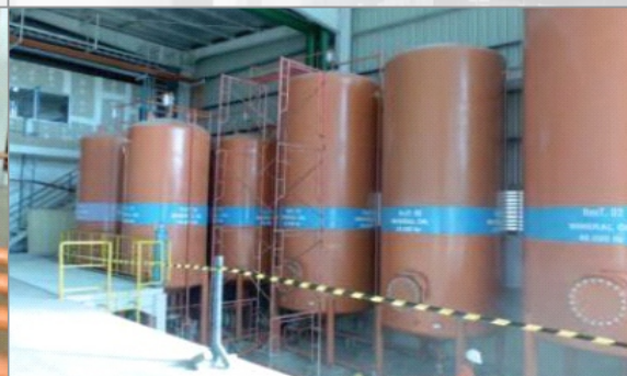
PIPING TANK AREA
