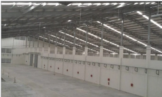
INSTALLATION LIGHTING HIGHBAY AREA FACTORY
