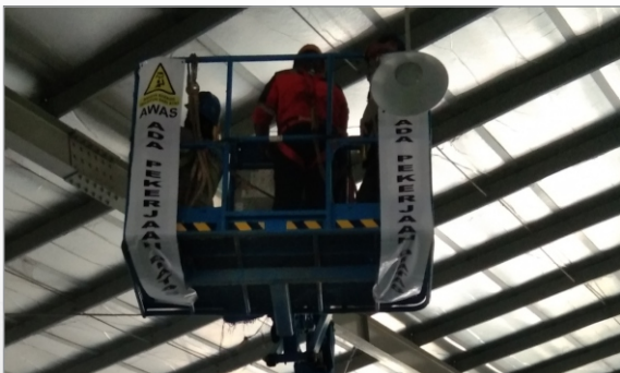
INSTALLATION LIGHTING AREA PRODUCTION
