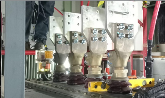
INSTALLATION CABLE TRAF0 2000 KVA
